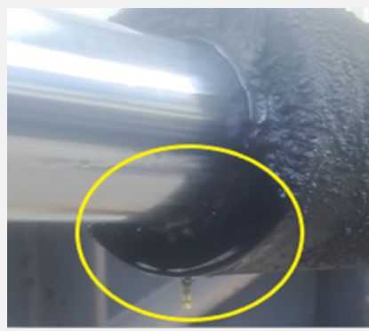
Major cylinder oil leak dripping oil
