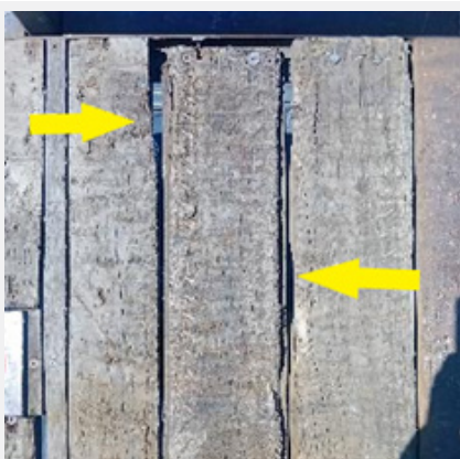
Worn & rotten deck planks with gaps
