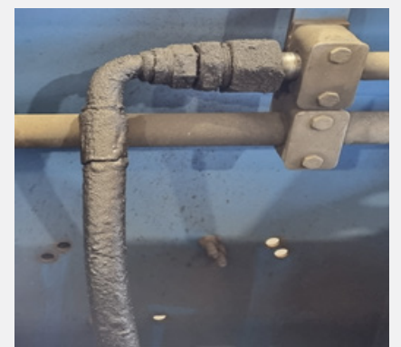
Leaking hydraulic hose
