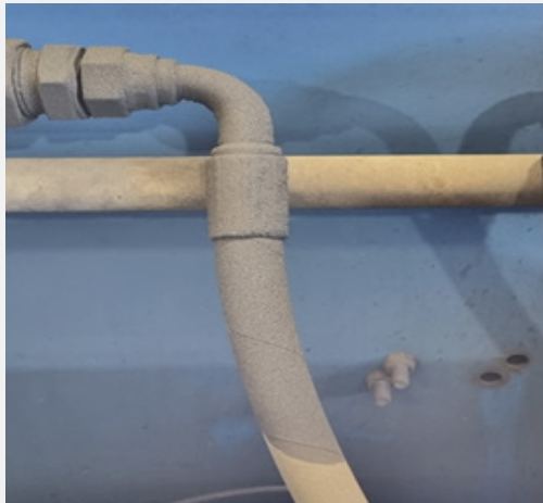
Minor misting on hydraulic hose
