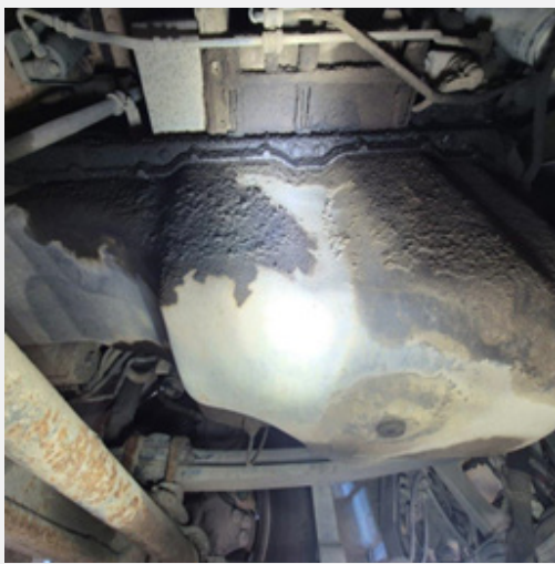
Engine oil leak requiring repair
